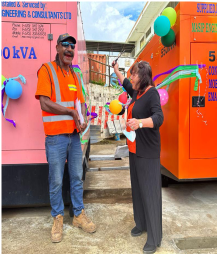
Picture Caption Massip Engineering and Consultant Ltd MD Timothy Kapak and PHA's acting CEO Jane Holden Officially launching 550KVA generator.
